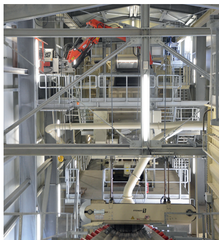
Primary crushing plant, raw gypsum, 400t/h, HAVER F-CLASS, apron conveyor, jaw crusher
