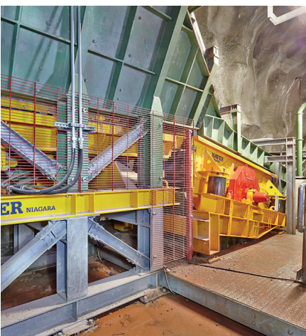
Primary crushing plant, fluorspar and feldspar, 80t/h, HAVER F-CLASS, HAVER push feeder, jaw crusher
