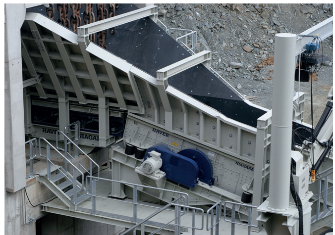
Rugged bunker construction using the HAVER reciprocating feeder
