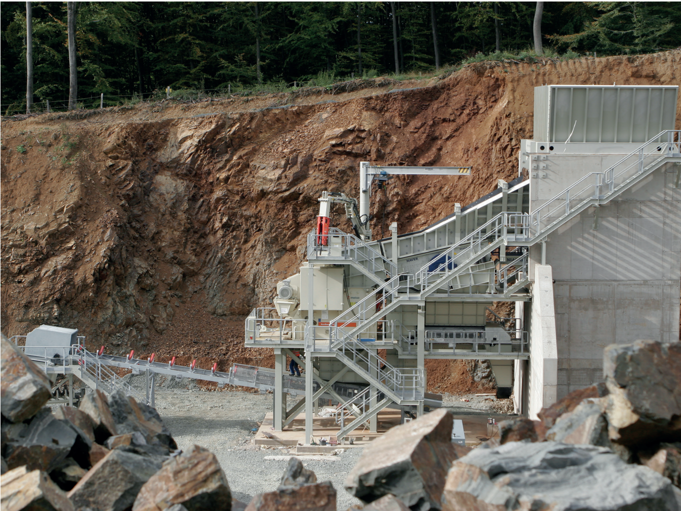
BASIC Primary crushing plant, diabase, 500t/h, HAVER F-CLASS, HAVER push feeder, jaw crusher
