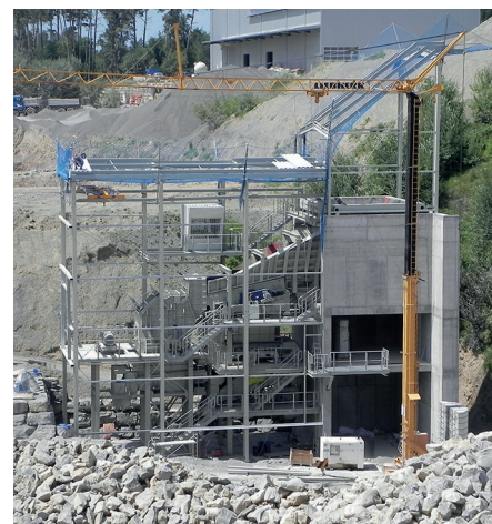
MASTER Primary crushing plant, limestone, 600t/h, HAVER F-CLASS, HAVER push feeder, impact crusher
