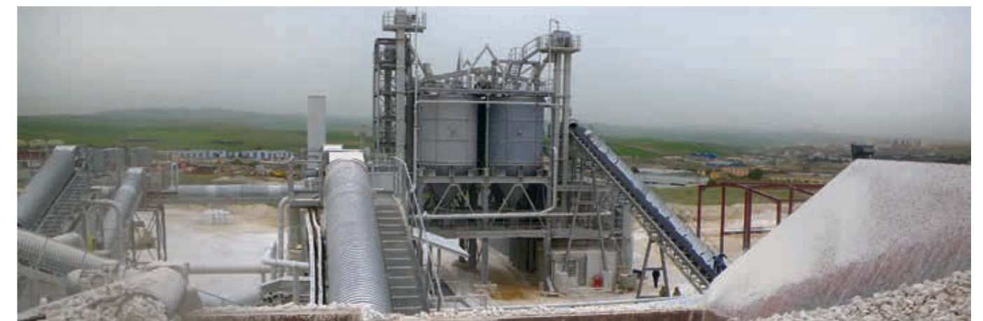
Primary crushing plant, calcium carbonate, 120t/h, HAVER vibrating feeder, cone crusher
