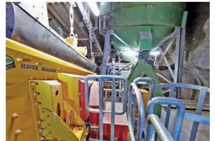
Primary crushing plant, fluorspar and feldspar, 80t/h, HAVER F-CLASS, HAVER push feeder, jaw crusher
