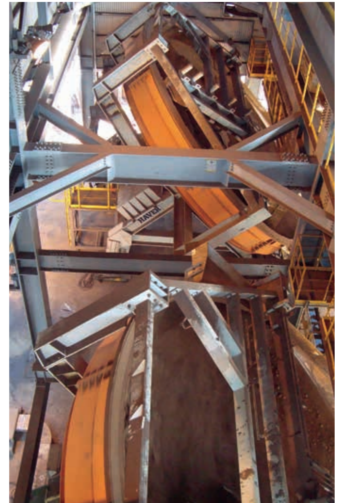
Pelletizing plant, iron ore, 140t/h, HAVER SCARABAEUS
